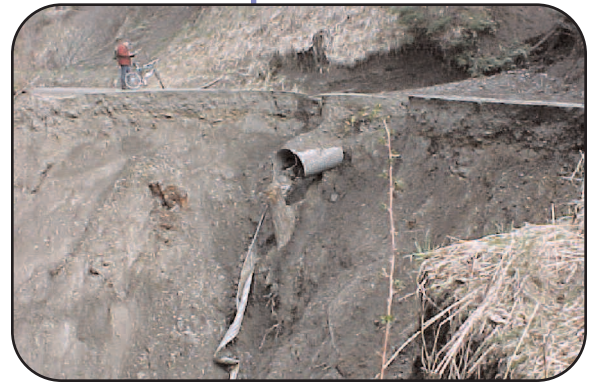
Extreme weather caused by climate change is likely to impact unmaintained roads. The runoff shown here threatens five threatened or endangered species of fish in the Olympic National Forest. (EPA PHOTO)
